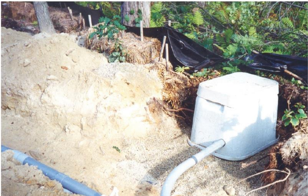
17.0-4 Properly Completed Transformer Installation (Final Grade)
